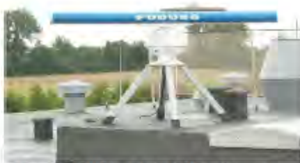
Figure 1: LAWR installation in Vejle, Denmark
