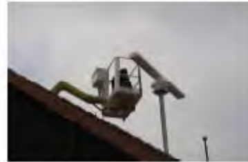
Figure 9: Installation in Hohensfels, Germany
