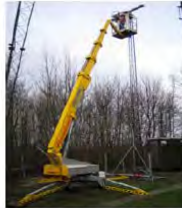
Figure 8: Installation at Søsterhøj, Denmark
