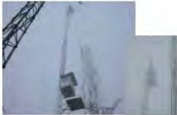
Figure 6: Installation in Ecuador The control unit is installed in the box, the radar itself on the top of the mast
