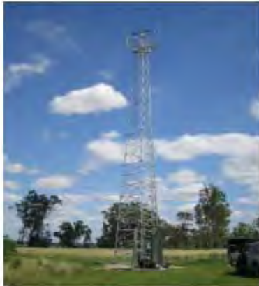
Figure 5: Installation in Toenda, Australia
